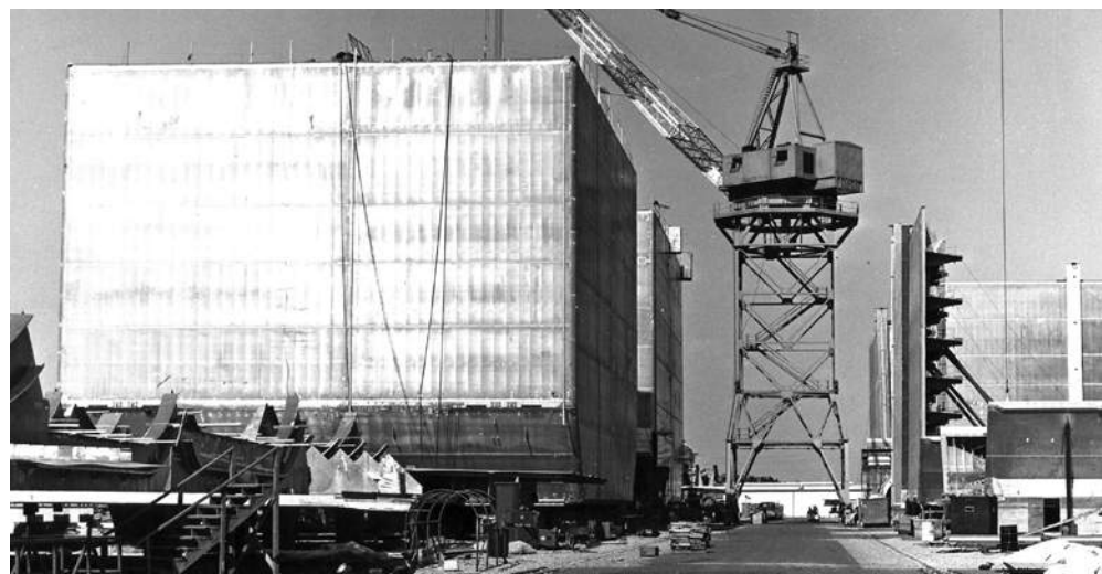
Conch prismatic tanks being assembled at Kaiser's Pinto Island facility in the late 1970s, for installation on the LNG carriers building at Avondale for El Paso
