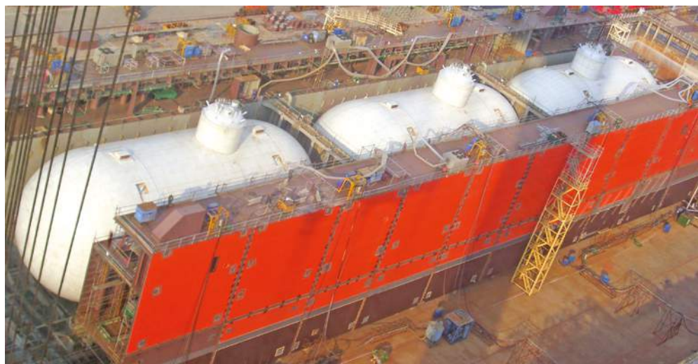
The FLNG Caribbean project is poised to show what is possible with small, barge-mounted liquefaction units
