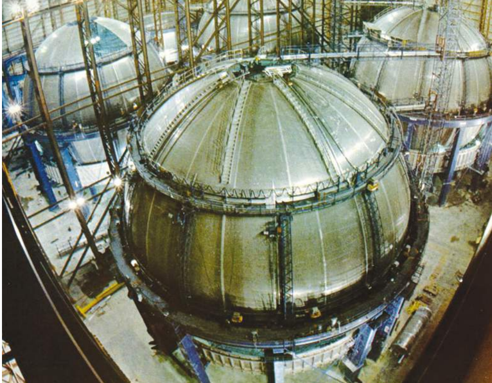
The assembly hall at Charleston, South Carolina enabled the simultaneous fabrication of up to six spherical tanks
