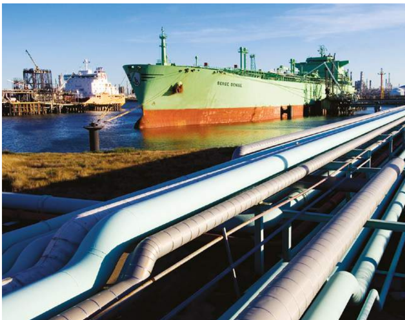
The Enterprise LPG export terminal in Houston has just completed one expansion project and is embarking on another
