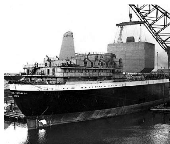
Methane Progress was fitted with nine self-supporting, prismatic tanks made of aluminium
